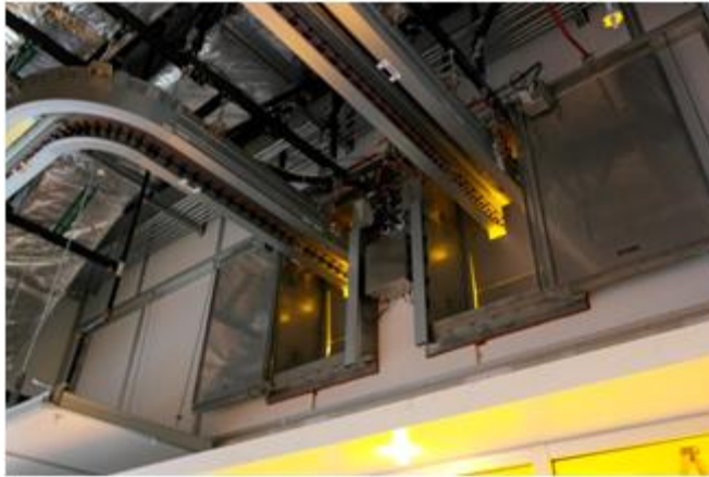
Figure 5. Fire Doors in NFX Link Area
