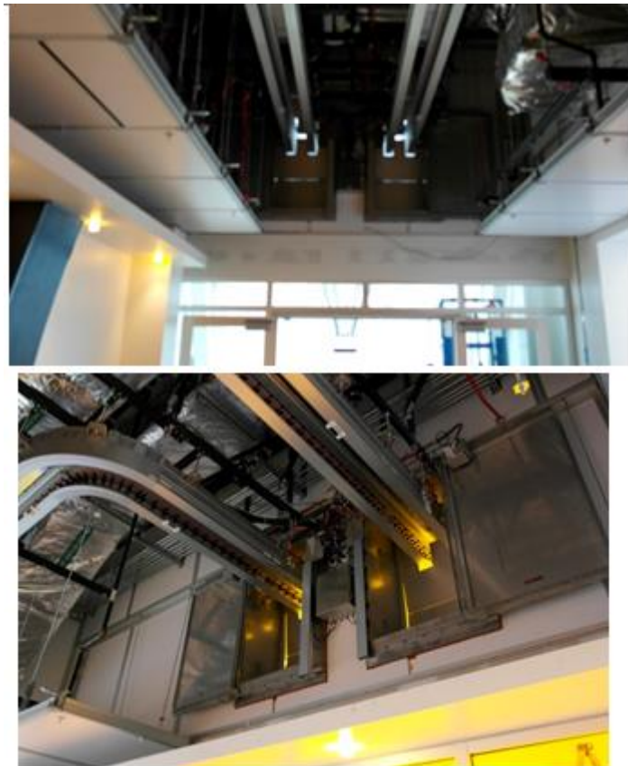
Figure 10 & 11. NFX Link Fire Door Set- Ceiling Tiles Removed
