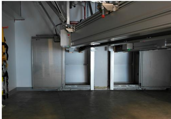
Figure 6. Fire Doors in NFN Tunnel Area
